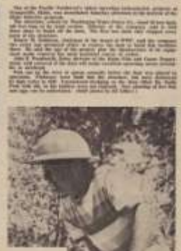
Demolition of the Washington Water Power Co. dam in active work at Grangeville, Idaho on the South Fork of the Clearwater River. The old structure was in
