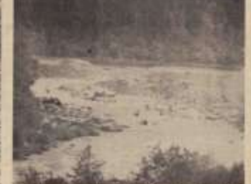
Demolition of the Washington Water Power Co. dam in active work at Grangeville, Idaho on the South Fork of the Clearwater River. The old structure was in
