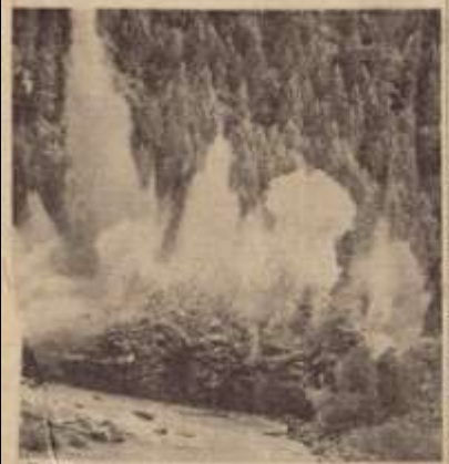
The blast of three dynamite blasts demolishing the Washington Water Power Co. dam in active work at Grangeville, Idaho on the South Fork of the Clearwater River. The old structure was in
