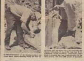
Demolition of the Washington Water Power Co. dam in active work at Grangeville, Idaho on the South Fork of the Clearwater River. The old structure was in
