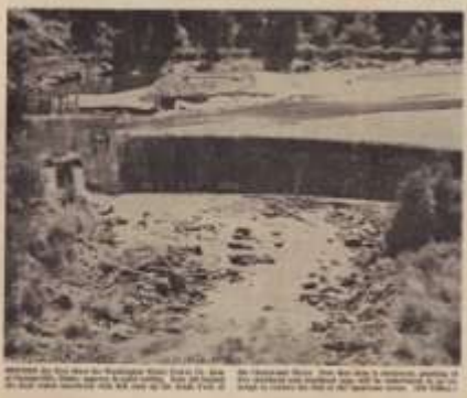
Demolition of the Washington Water Power Co. dam in active work at Grangeville, Idaho on the South Fork of the Clearwater River. The old structure was in
