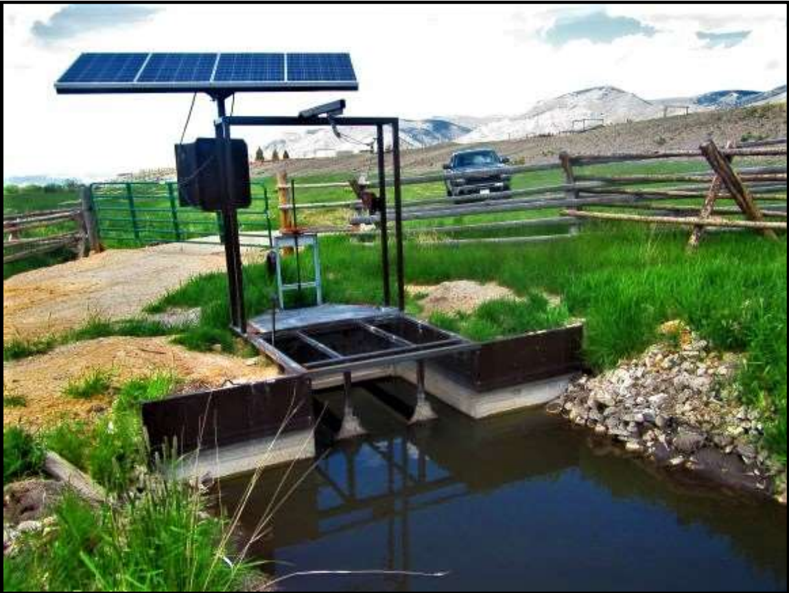
Photo 12. New NMFS criteria fish screen installed at the Eighteenmile Creek-01 (LEM-01) diversion in 2018.
