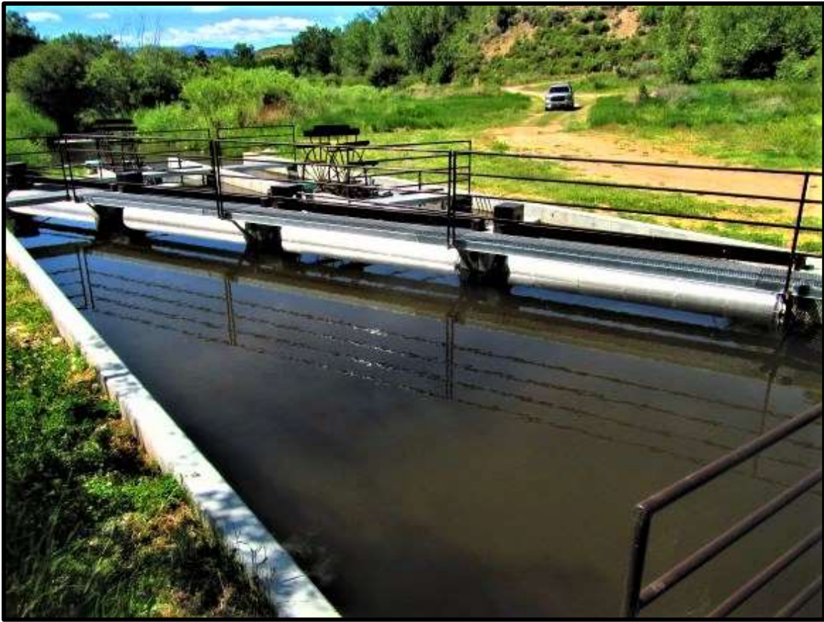
Photo 1. The Lemhi River-08A (L-08A) fish screen was replaced with a new and larger screen that was installed in fall of 2017.
