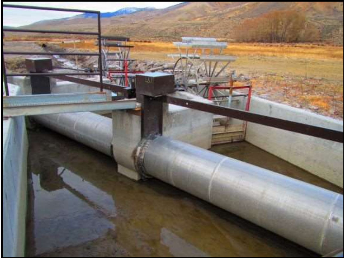
Photo 9. A new NMFS Criteria fish screen is replacing a fish screen that was not functioning properly due to age and poor drainage. The concrete was poured and screen fabricated in 2018, but the screen will not be completed until the headgate and ditch works are installed in summer of 2019.
