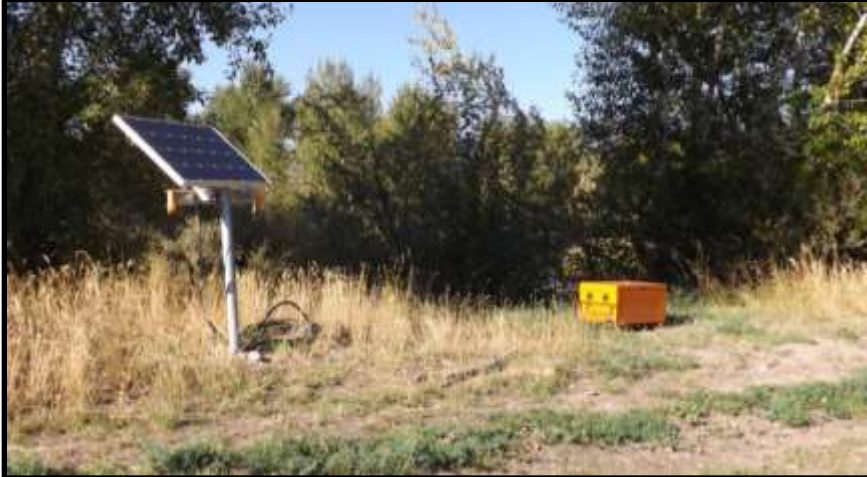
Photo 18. Solar and battery power installed to power the new PIT tag detection systems purchased in 2015.
