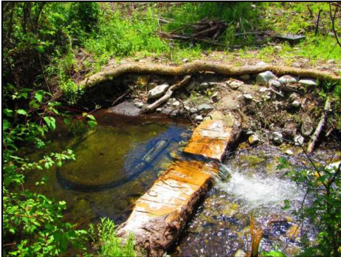
Photo 10. Pratt-Hedt passive fish screen was installed in December 2018. The screen and hose will need to be seasonally removed by the irrigator.
