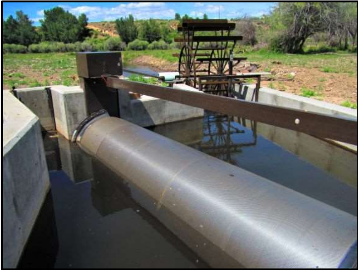
Photo 16. New NMFS Criteria fish screen installed at L-03AO is replacing a fish screen that was not functioning properly due to age and poor drainage.
