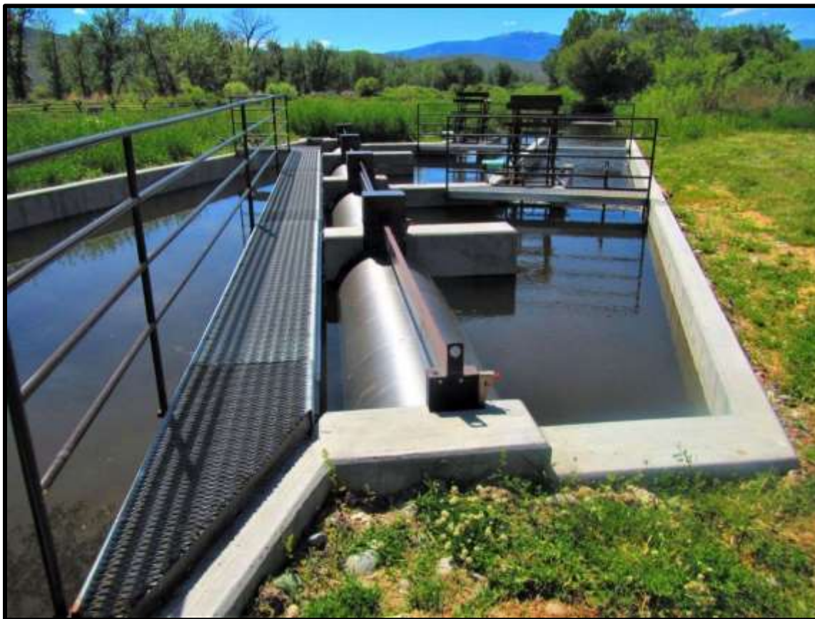
Photo 13. The metal works of the L-08A fish screen was installed in spring of 2018.
