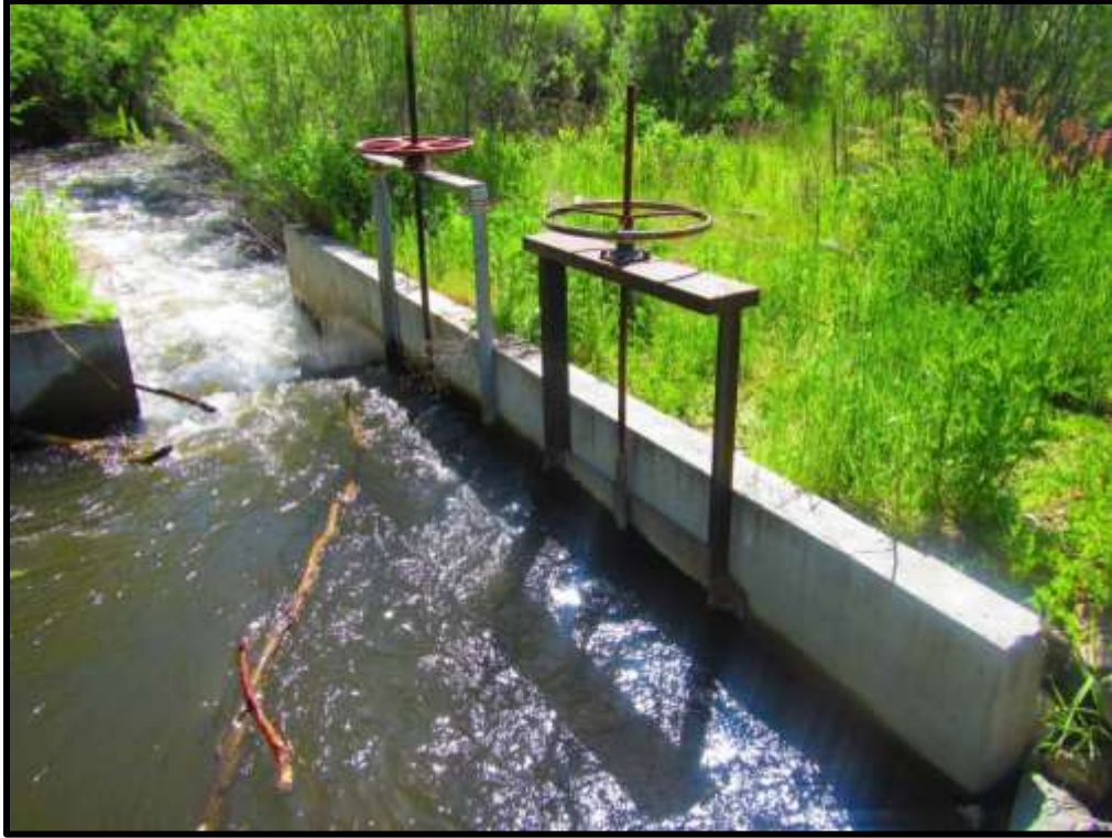
Photo 14. A second headgate was installed to accommodate the additional 18 CFS of water needed to complete the flow projects.
