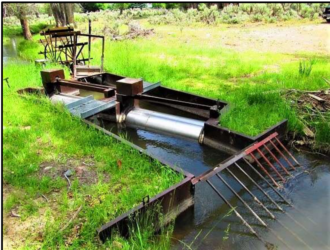
Photo 6. New NMFS criteria fish screen installed at the Salmon River-23A (S-23A) diversion in 2017.
