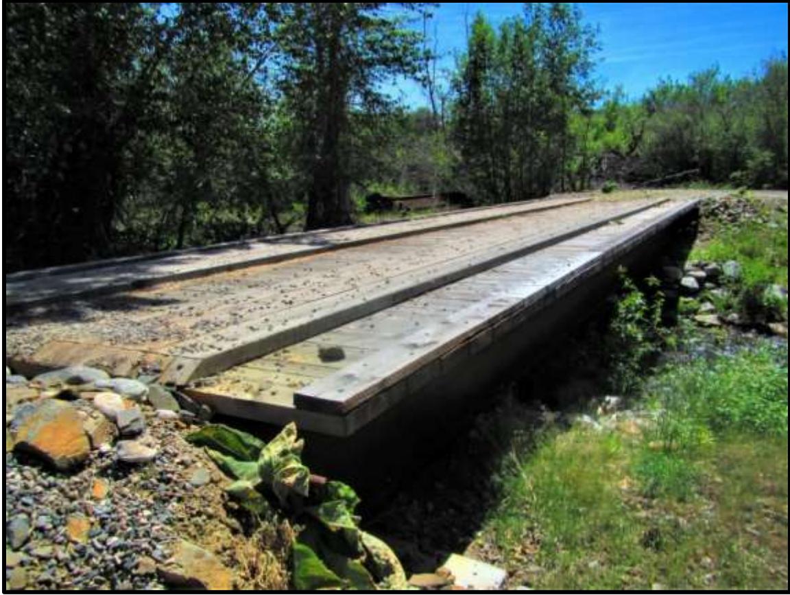
Photo 8. The old Carmen Creek -03 (SCC-03) access bridge was replaced with a new bridge in January 2018.
