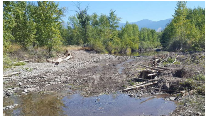
Constructed riffle during construction; LWM bank structure installed on left bank (right side of photo) to reduce over-widened channel width; Lemhi River, ID
