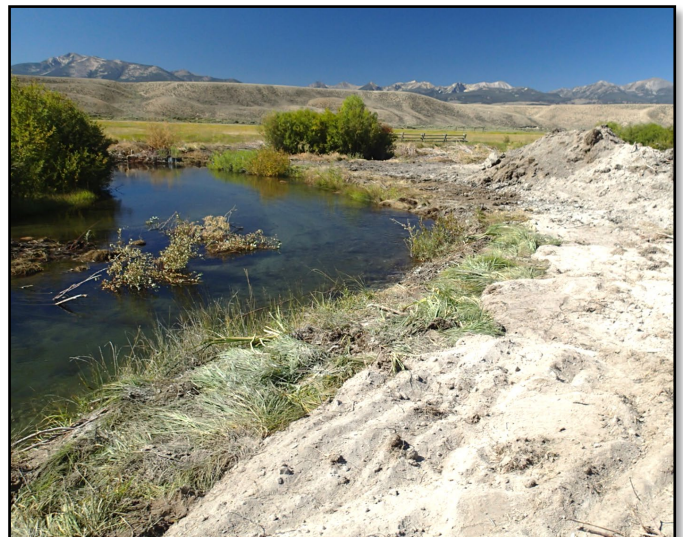
Thick strips of wetland sod harvested on-site used to retain unstable sandy bank fill immediately after construction; Big Springs Creek, ID
