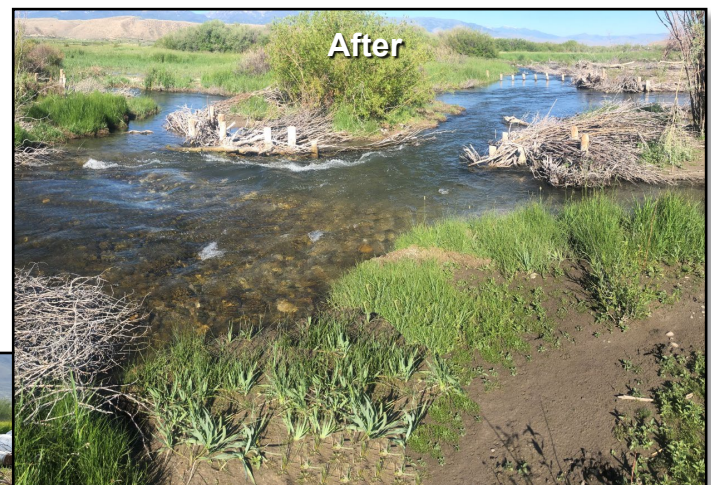
Lemhi River, 1.5 years after construction of multi-threaded channel network using various bank treatments and instream structure to split flow into many, short, narrow side channels; average width less than 20 ft.
