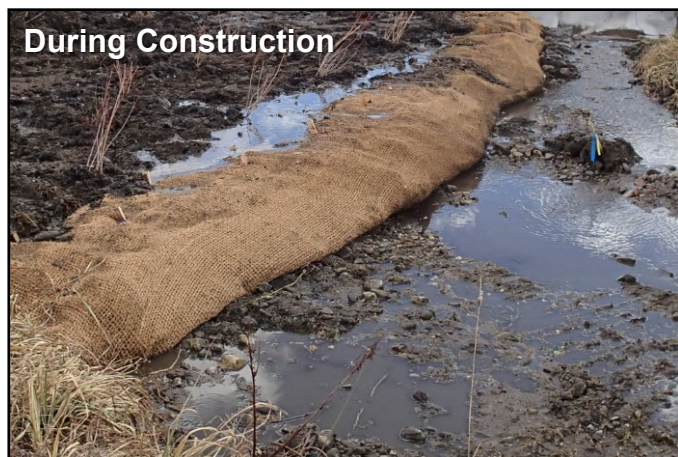
Big Springs Creek during construction; Fill placed behind the FESL with potted plants; Sod mat and potted plants within FESL not yet installed
