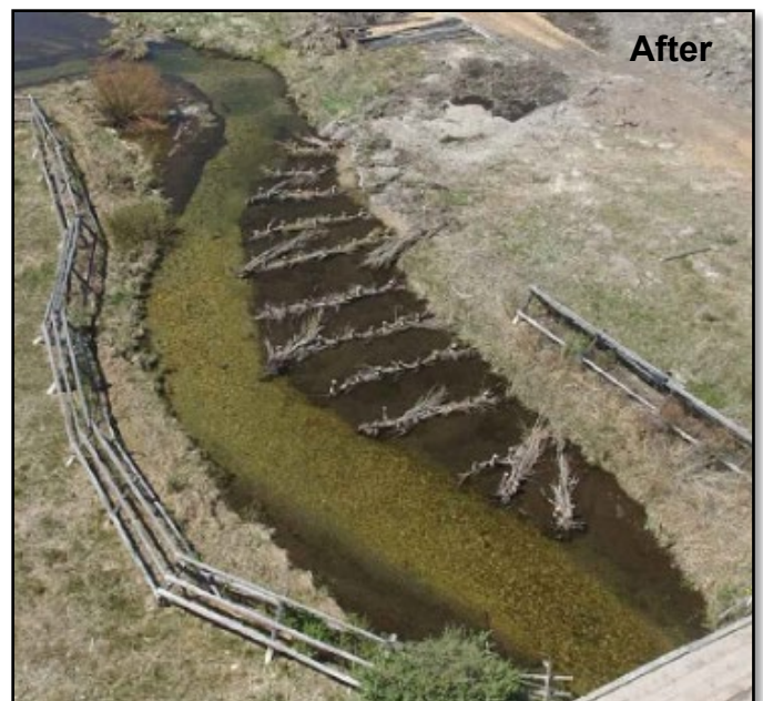
6 months after construction; fine sediment deposition observed between willow weaves; effective channel width reduced by approximately 50%
