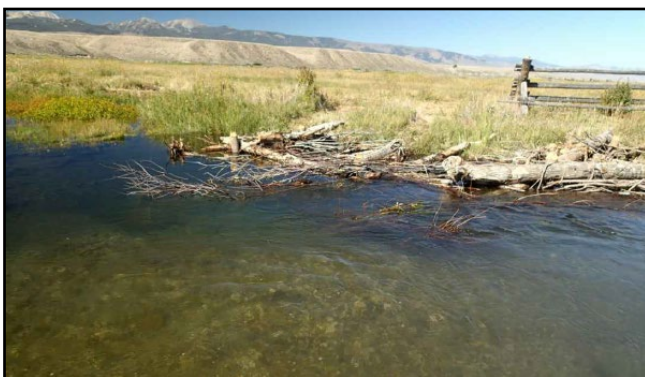
Small wood material bank structures with excavated scour pool immediately after construction; Big Springs Creek, ID
