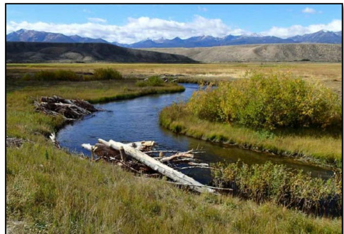
Small and large wood material bank structures immediately after construction; Big Springs Creek, ID
