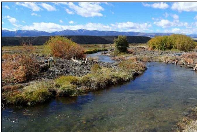
Bank fill stabilized with on-site harvested wetland sod immediately after construction; Big Springs Creek, ID
