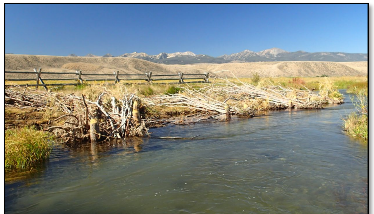
Series of willow clumps placed along the outside of a newly constructed meander bend to provide bank stability, instream structure, and cover immediately after construction; Big Springs Creek, ID
