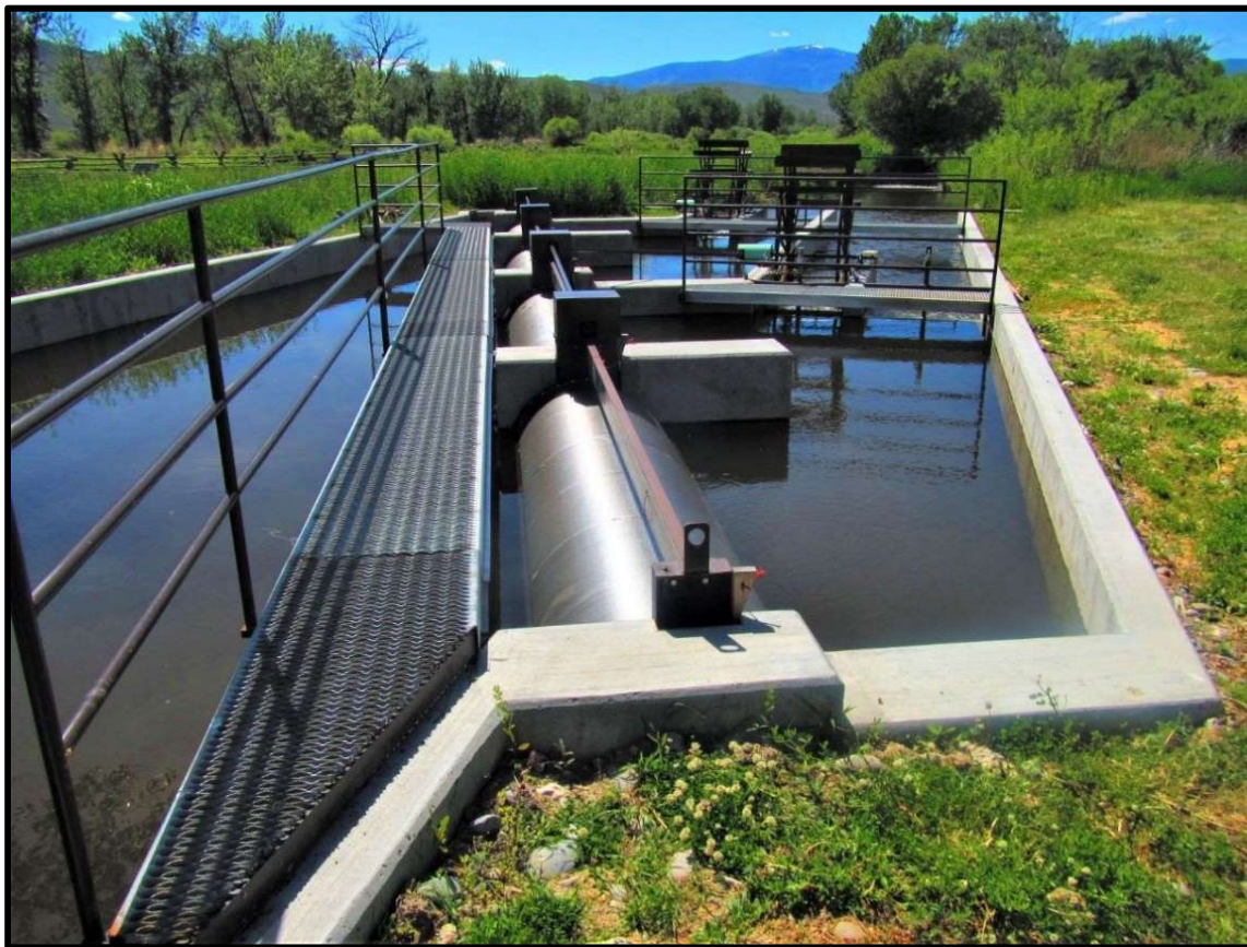
Photo 67. The metal works of the L-08A fish screen was installed in spring of 2018.
