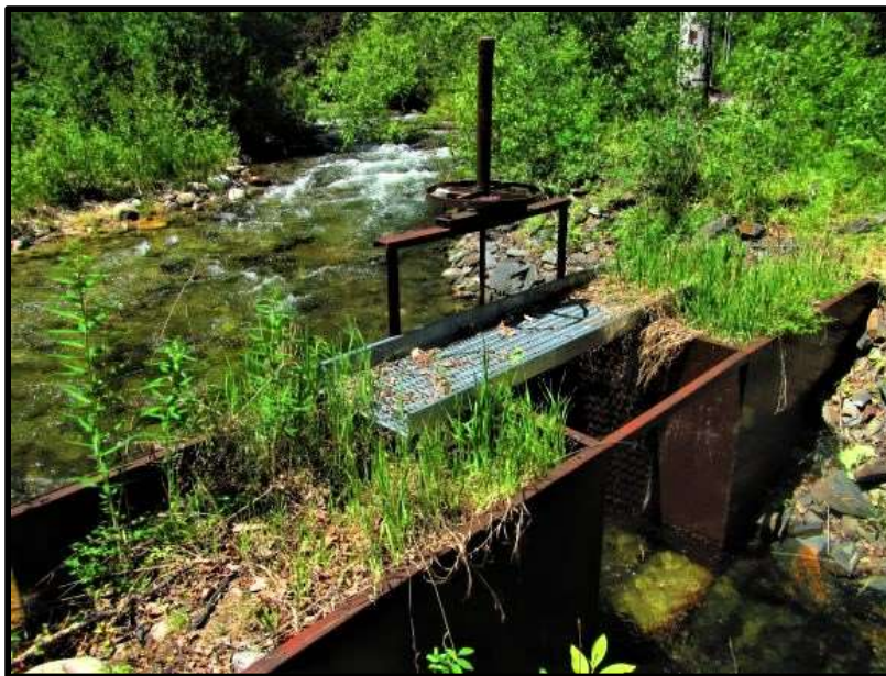
Photo 8. —New diversion and headgate installed to improve fish passage on Carmen Creek.
