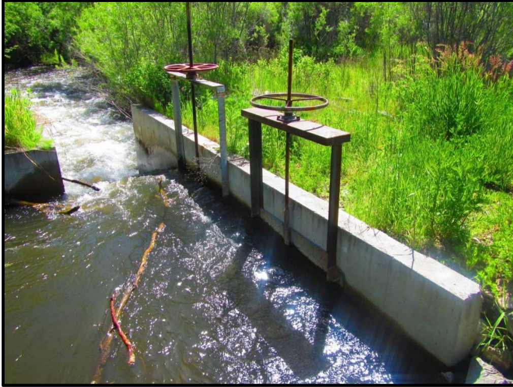
Photo 68. A second headgate was installed to accommodate the additional 18 CFS of water needed to complete the flow projects.
