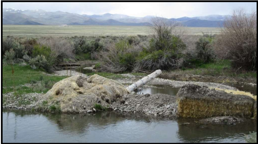
Photo 36. —The old P-16 diversion seasonally dewatered the Pahsimeroi River and was a barrier to fish passage.
