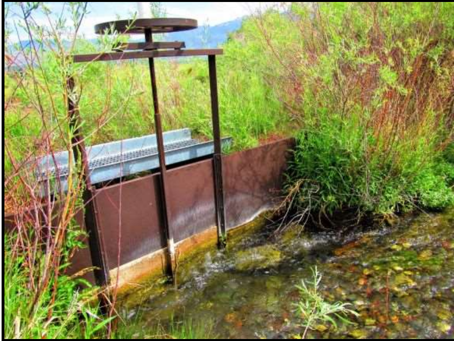
Photo 3. —New diversion and headgate were installed on Sulphur Creek-01 (PSC-01) diversion in 2014.
