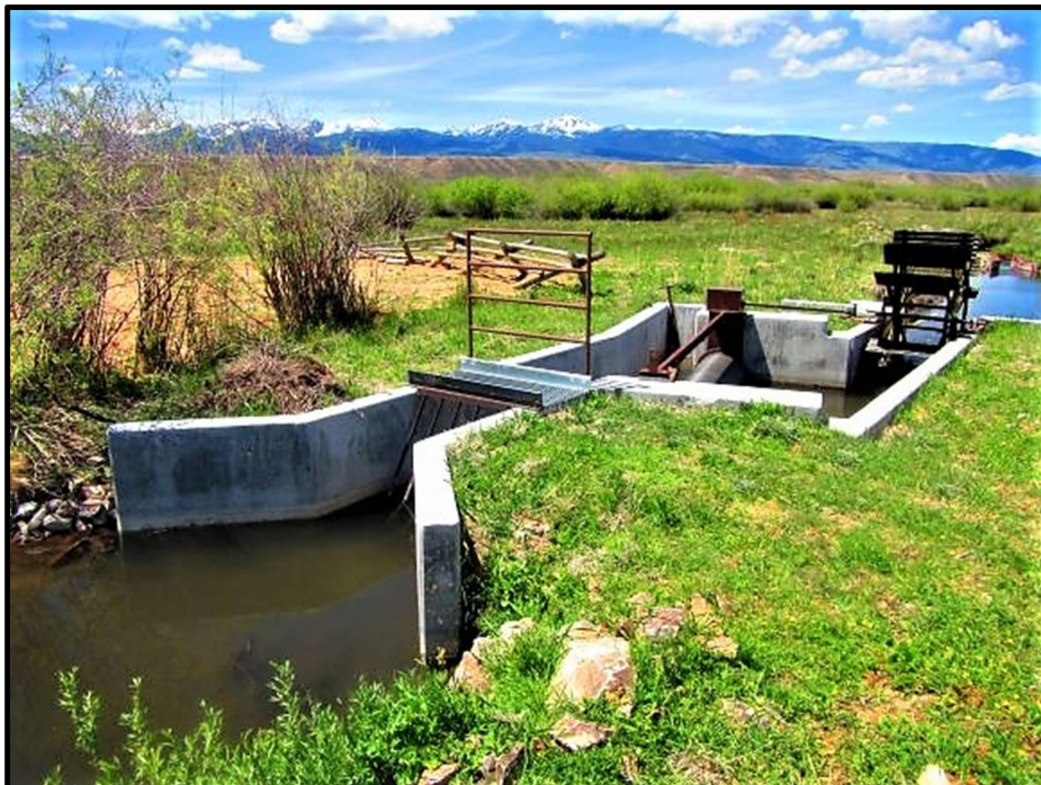
Photo 60. —New concrete installed at the Lemhi River (L-60) diversion in 2017. The metal works and screen were fabricated in the Screen Shop and installed to NMFS criteria.
