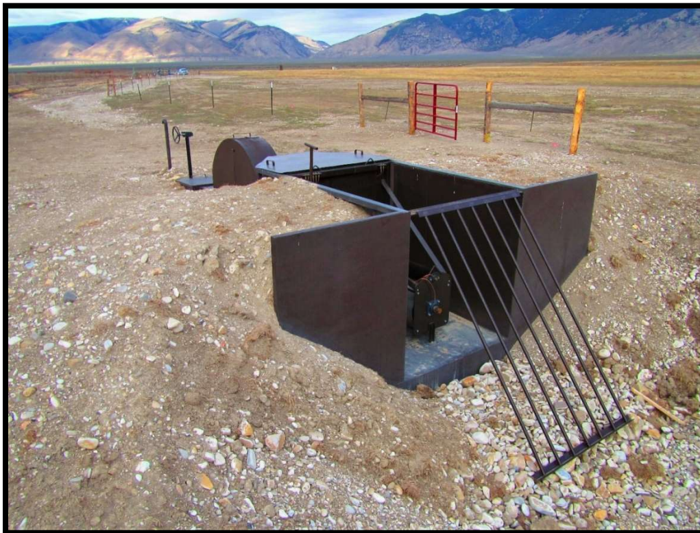
Photo 79. A new NMFS Criteria fish screen was installed on the Eighteen Mile Creek-Breshears (LEMC-03) at the Breshears property. This screen will be in service next spring for irrigation season.
