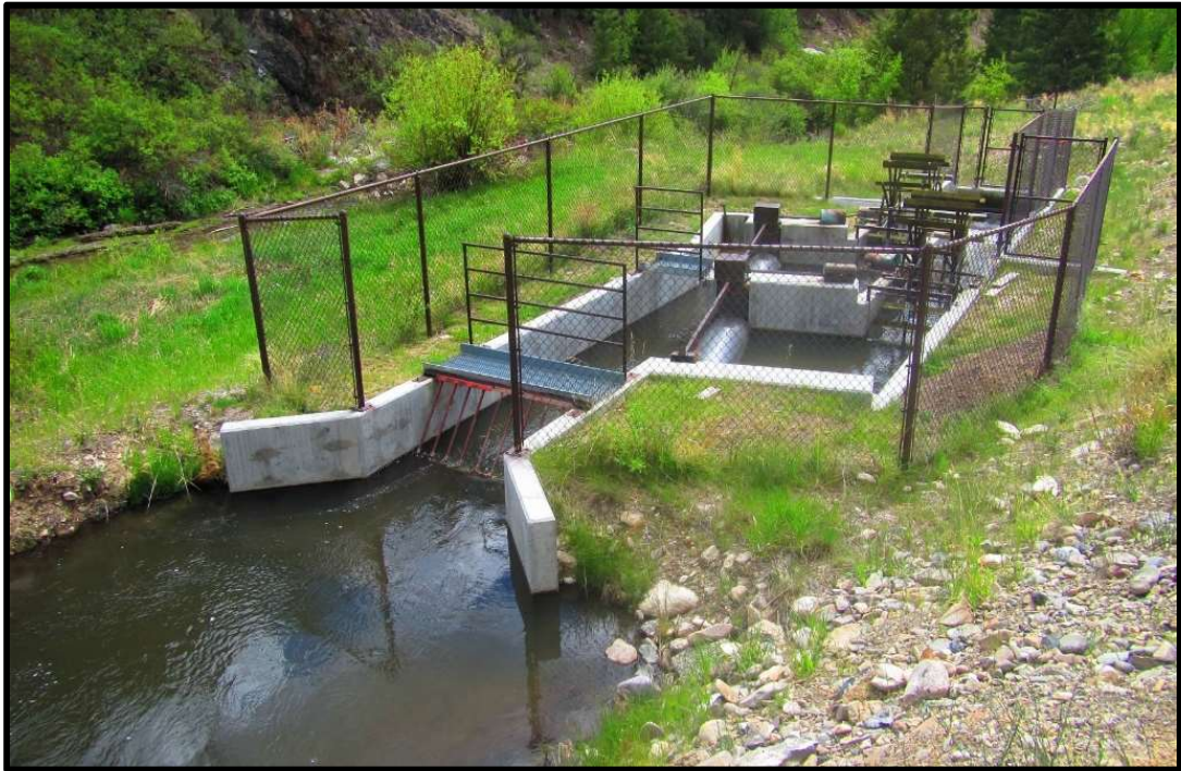
Photo 20. —New NMFS criteria fish screen was installed on the Hawley Creek-03 diversion in 2014. The screened water now enters a closed pipeline irrigation system resulting in water savings of 5.2 CFS for instream flow.
