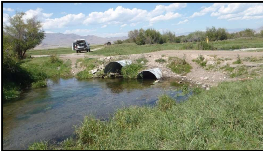
Photo 13. —Patterson Big Springs ranch road crossing was a fish passage barrier.
