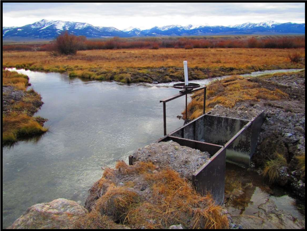
Photo 76. A new headgate was installed and the channel was rerouted into a newly constructed stream channel at L-61.
