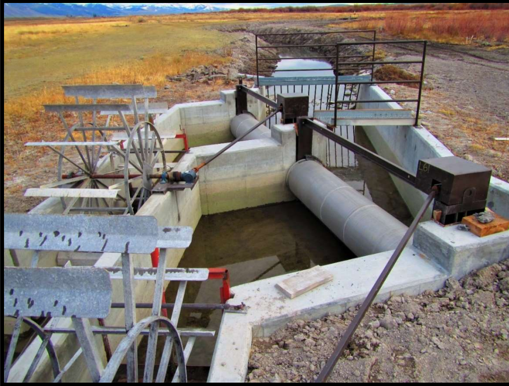
Photo 77. A new NMFS Criteria fish screen replaced a fish screen that was not functioning properly due to age and poor drainage. The concrete was poured and screen fabricated in 2018, but the screen was completed when the headgate and ditch works were installed in summer of 2019.
