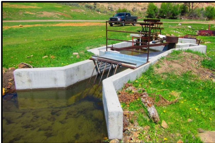
Photo 30. —New NMFS criteria fish screen installed at the Hayden Creek-08 diversion in 2014.
