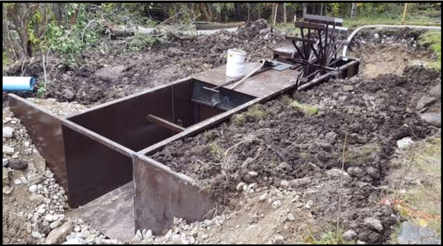
Photo 56. —The Pratt Creek-01 fish screen was installed as part of a water savings, fish passage, and screening project. The site will be reclaimed and re-seeded fall 2016 or spring of 2017.
