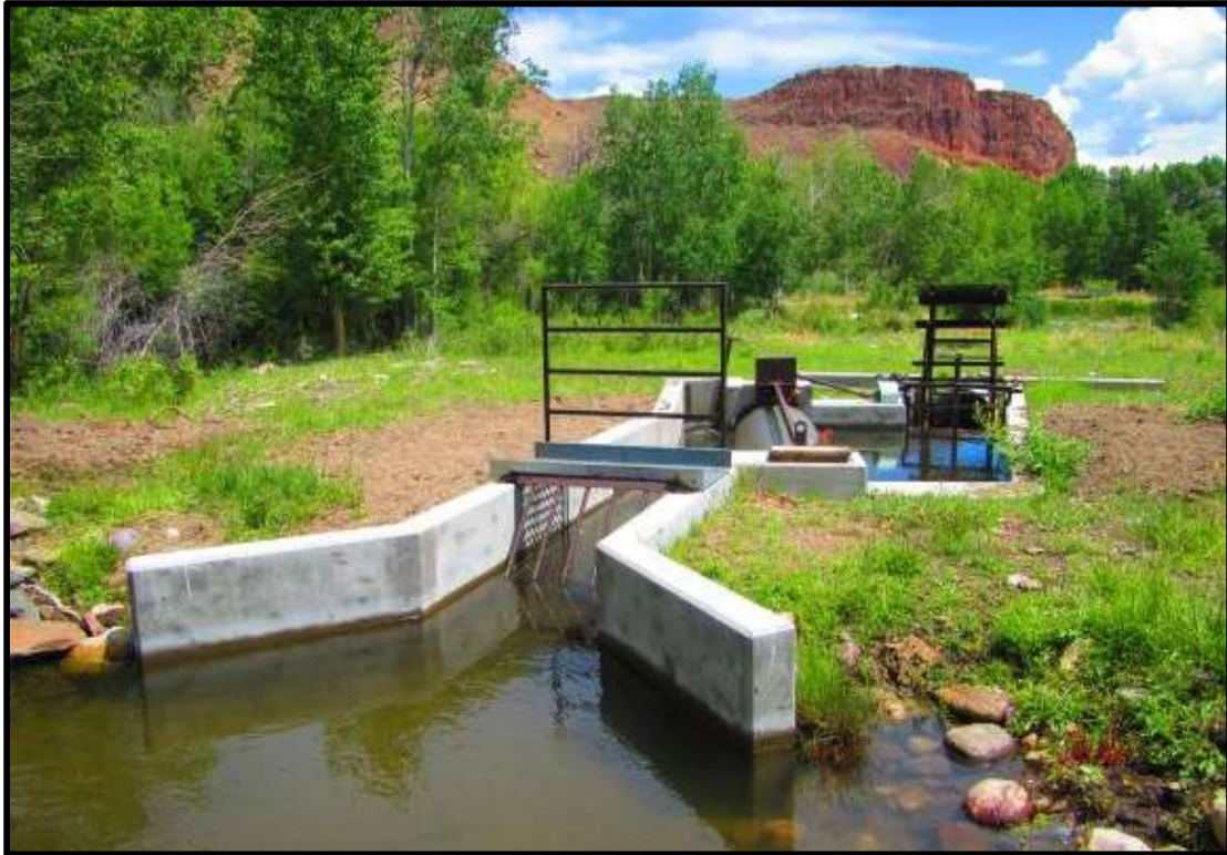
Photo 42. —New NMFS criteria fish screen installed at the Garden Creek-01 diversion in 2015.
