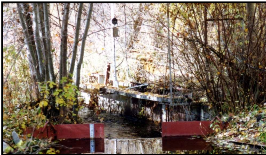
Photo 43. —Wiper screen on Carmen Creek-03 diversion before replacement.
