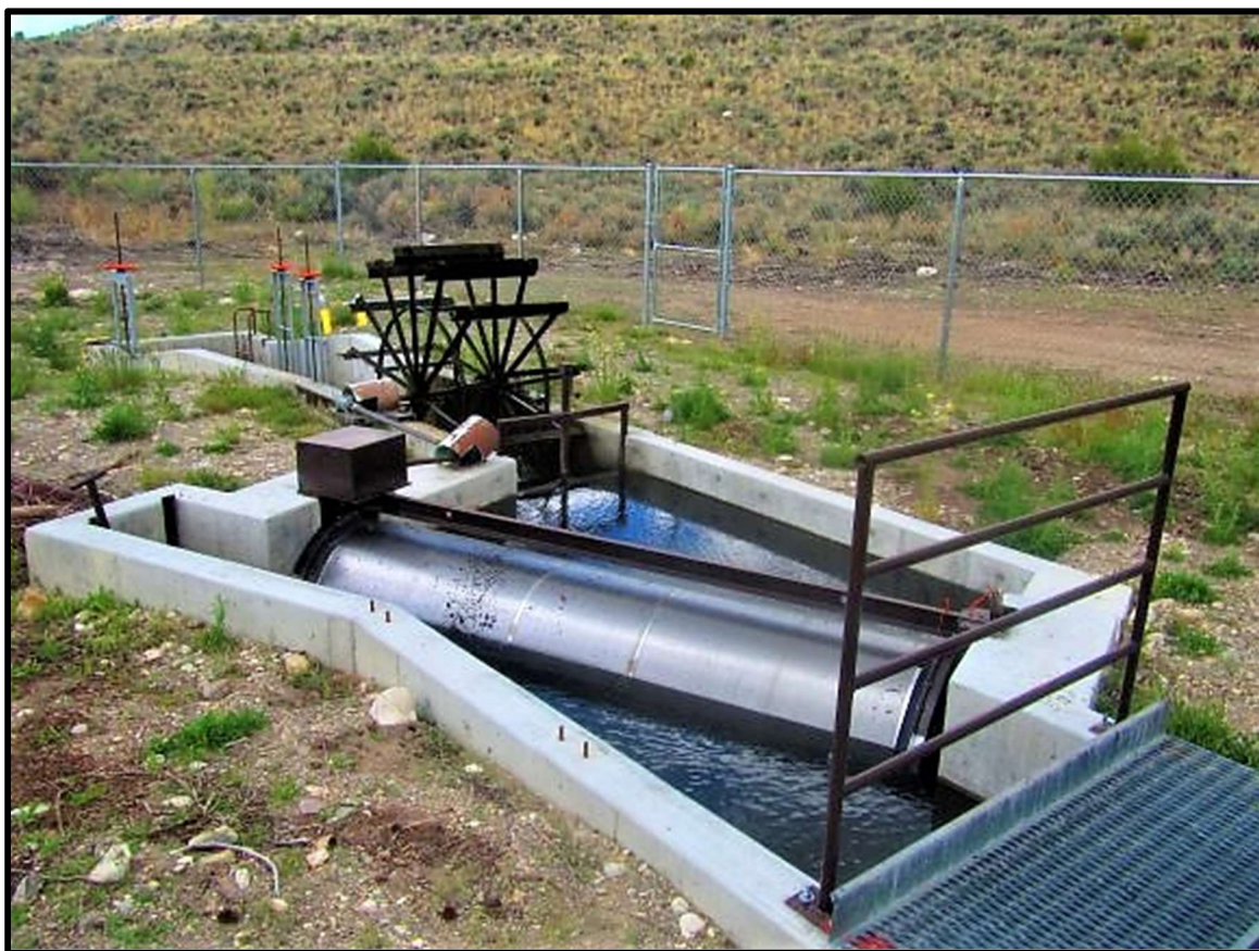
Photo 58. —New NMFS criteria fish screen installed at the Hawley Creek (LHaw-02) diversion in 2017.
