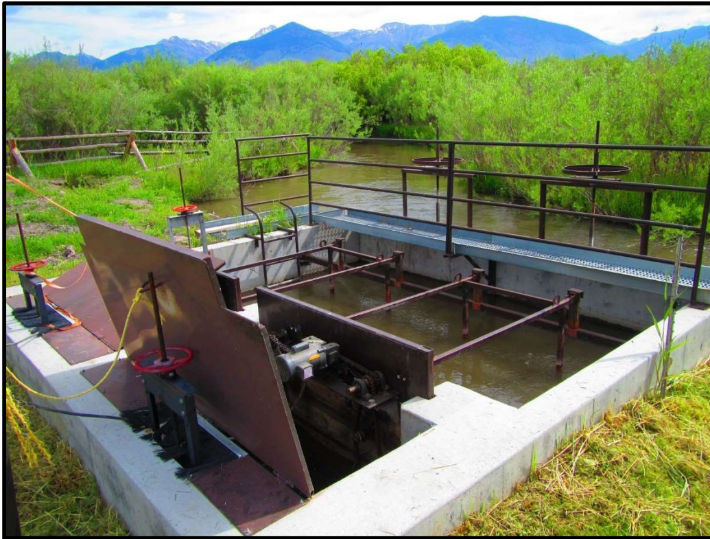
Photo 25. —New NMFS criteria fish screen and diversion was installed at the Pahsimeroi-13 Pump Station in 2014 and flow and fish passage was restored to this reach of river.
