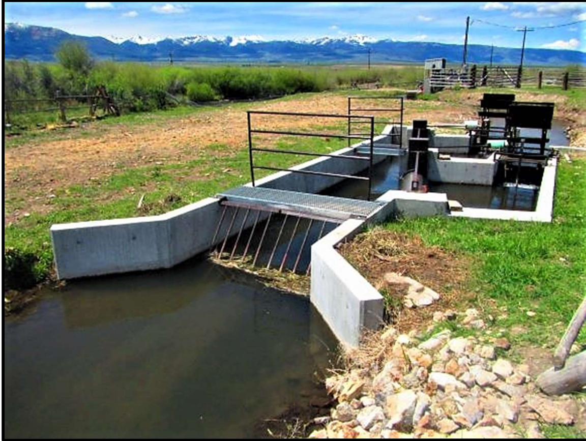
Photo 61. —New concrete installed at the Lemhi River (L-62) diversion in 2017. The metal works and screen were fabricated in the Screen Shop and installed to NMFS criteria.
