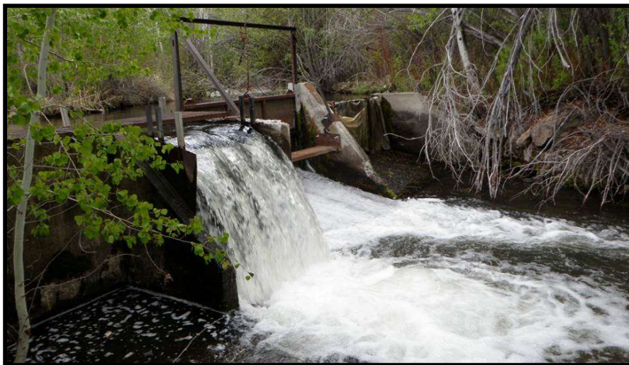
Photo 39. —Garden Creek-01 diversion was a fish barrier before replacement.
