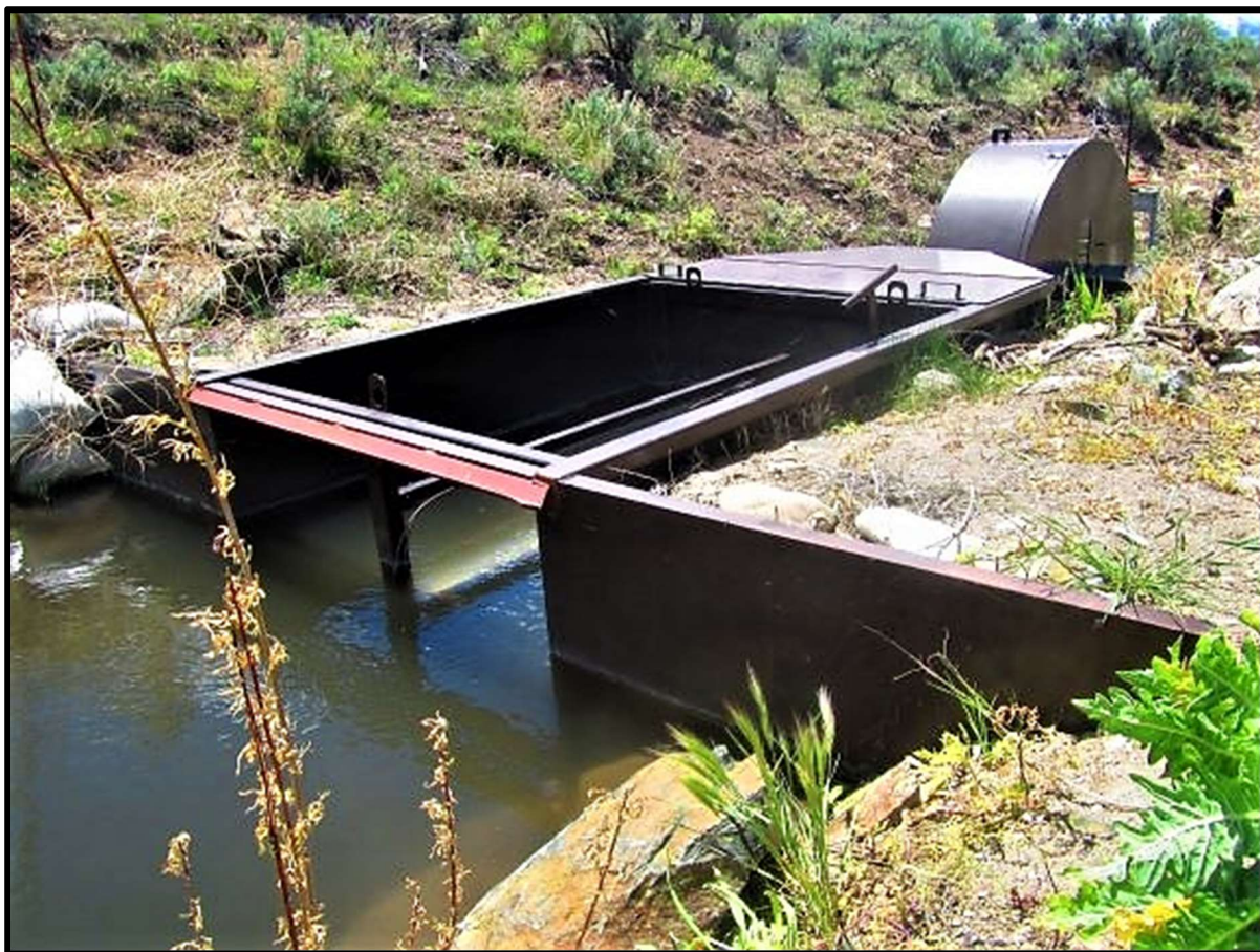
Photo 59. —New NMFS criteria closed drum fish screen installed at the Canyon Creek (LCanyC-03) diversion in 2017.
