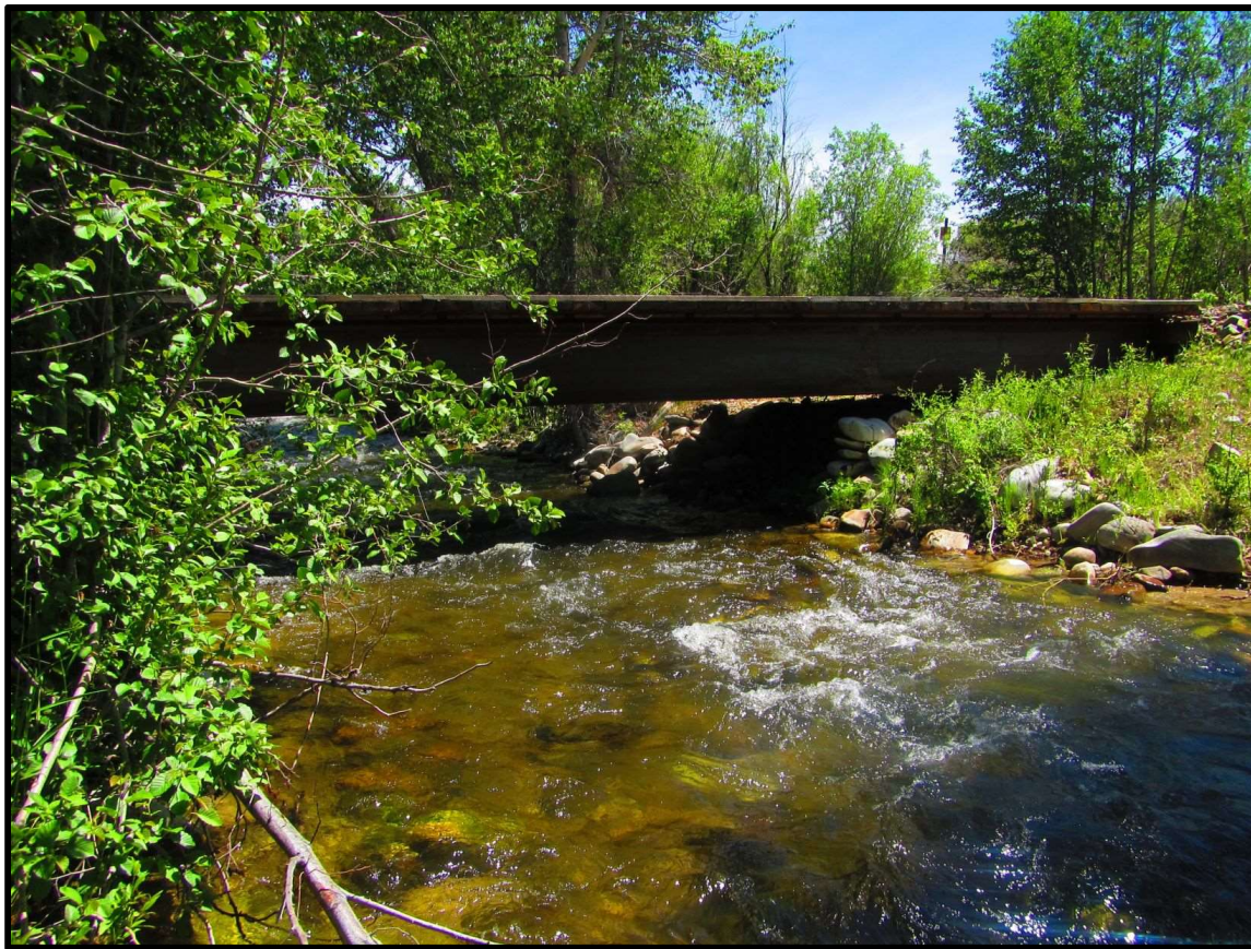
Photo 63. The old Carmen Creek -03 (SCC-03) access bridge was replaced with a new bridge in January 2018.
