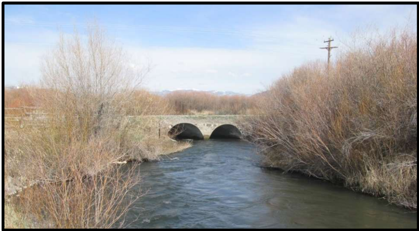
Photo 52. —Undersized culvert across the Pahsimeroi River at Dowton Lane was a partial barrier to fish passage.
