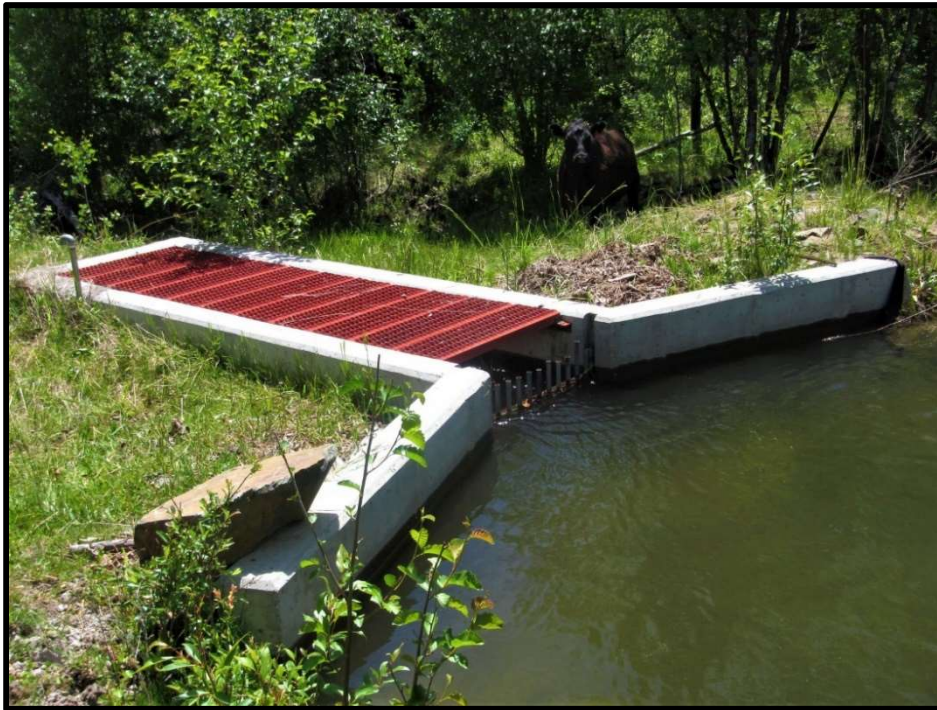
Photo 10. —A pipeline and siphon were installed to move the diverted water under Carmen Creek back to the point of use downstream.
