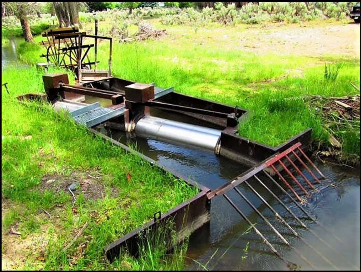
Photo 62. —New NMFS criteria fish screen installed at the Salmon River (S-23A) diversion in 2017.
