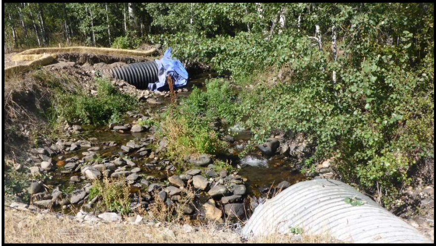
Photo 48. —Undersized culvert across Bohannon Creek was a partial barrier to fish passage.
