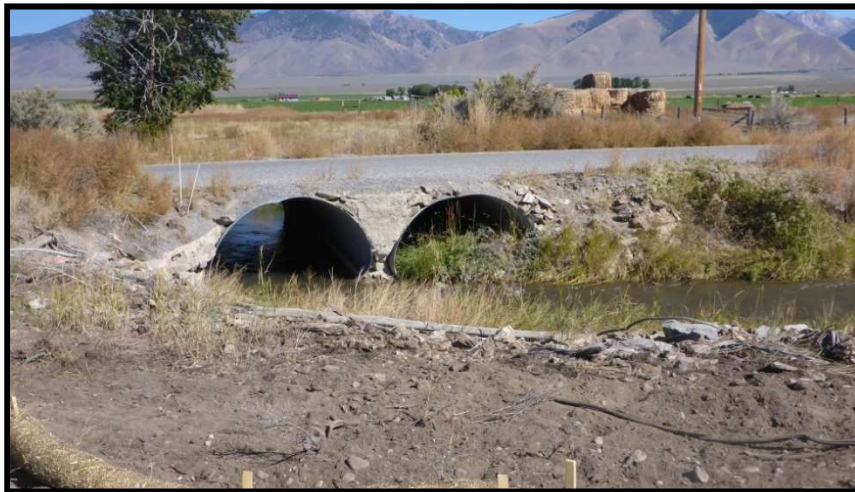
Photo 50. —Undersized culvert across the Pahsimeroi River at Furey Lane was a partial barrier to fish passage.
