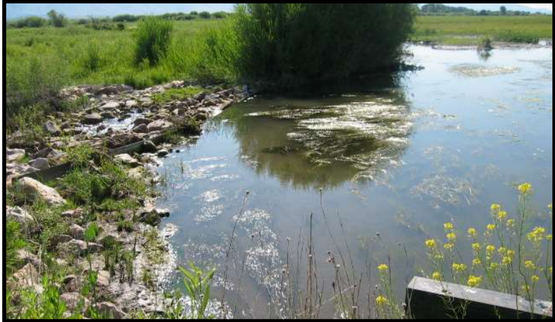
Photo 24. —Before the implementation of this project, the P-13 diversion created a fish passage barrier for both Sulphur Creek and the Pahsimeroi River.
