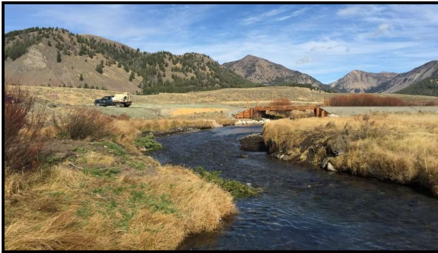
Photo 35. —The old Pole Creek-01 diversion was removed and the site was reclaimed in October 2015.
