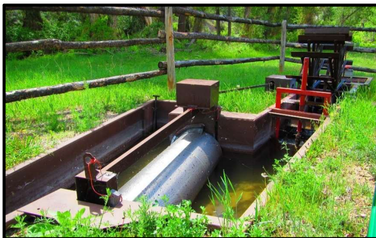
Photo 28. —New NMFS criteria fish screen was installed on the Poison Creek-01 diversion in 2014.
