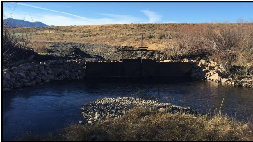
Photo 33. —A new headgate and ditch were installed at the new Pole Creek-01 point of diversion.
