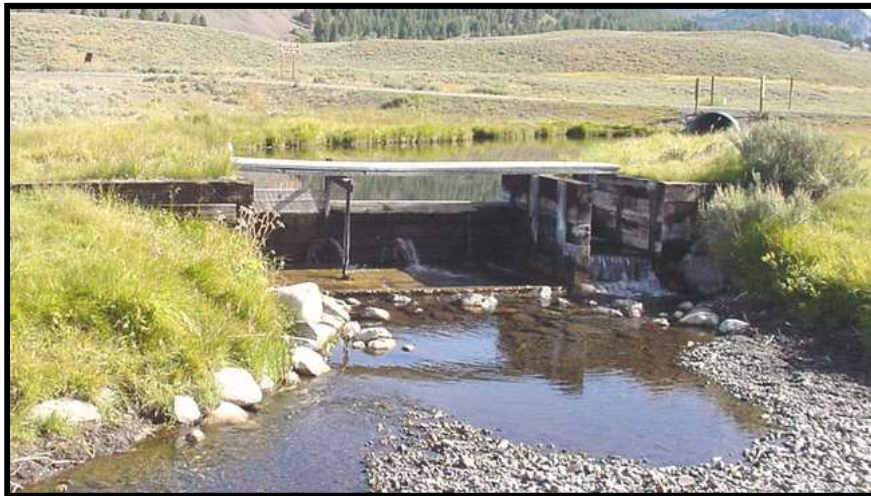
Photo 31. —The old Pole Creek-01 diversion seasonally dewatered Pole Creek and was a barrier to fish passage.
