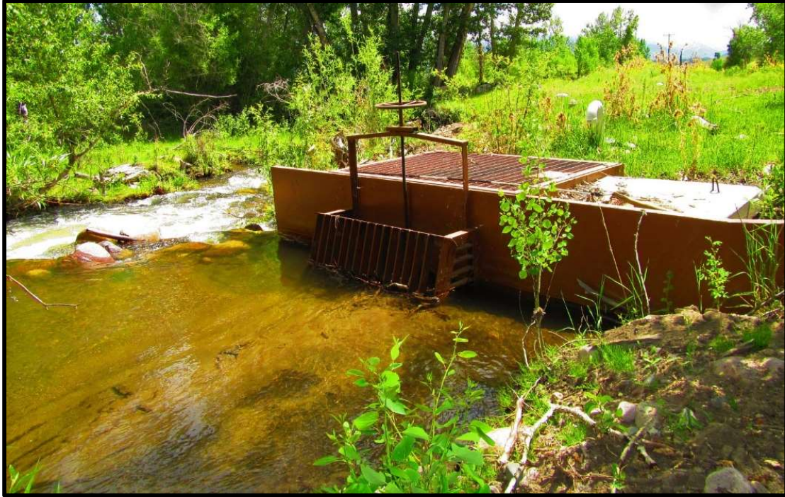
Photo 41. —New headgate controls water withdrawal on the Garden Creek-01 diversion.
