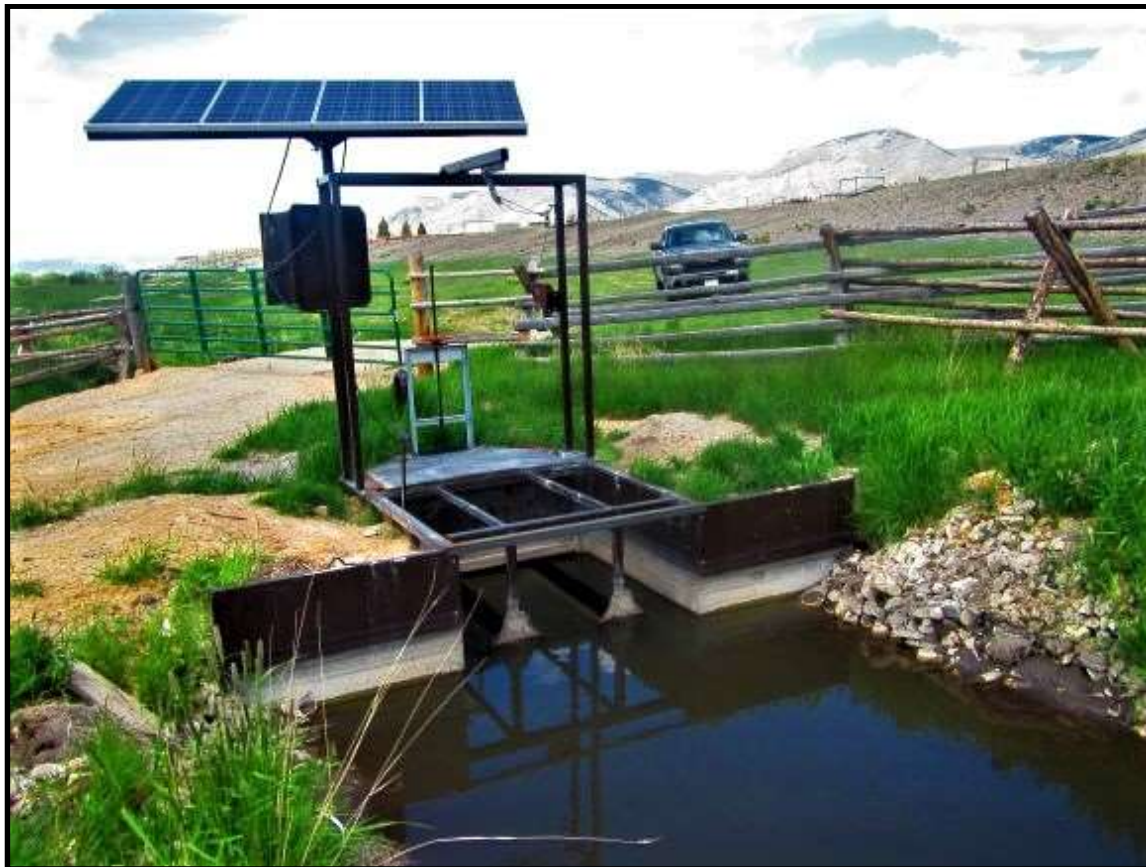
Photo 66. New NMFS criteria fish screen installed at the Eighteen Mile Creek-01 (LEM-01) diversion in 2018.
