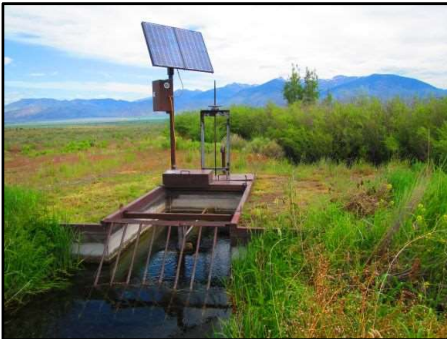
Photo 4. —New NMFS criteria fish screen was installed on the Sulphur Creek-01 diversion in 2013. The screened water now enters a closed pipeline irrigation system resulting in water savings of 4.5 CFS for instream flow.
