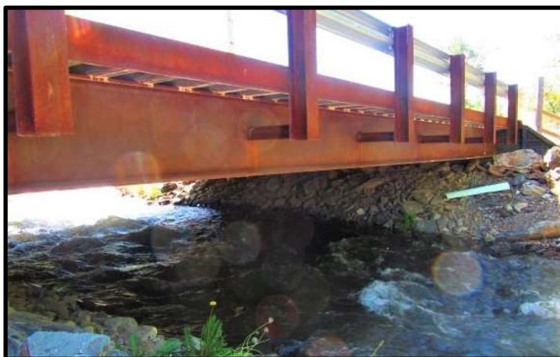
Photo 16. —New bridge across Wimpey Creek was installed in 2013 to eliminate a culvert passage barrier.
