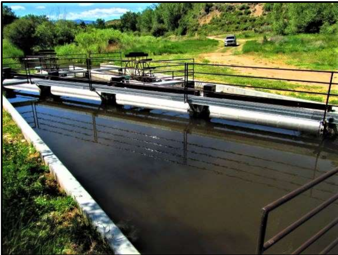
Photo 57. —New concrete installed at the Lemhi River (L-08A) diversion in 2017. The metal works and screen were fabricated in the Screen Shop and installed to NMFS criteria.
