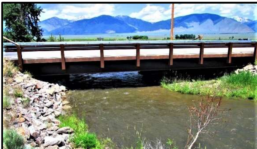
Photo 51. —New bridge across the Pahsimeroi River at Furey Lane was installed in 2015 to eliminate a passage barrier.
