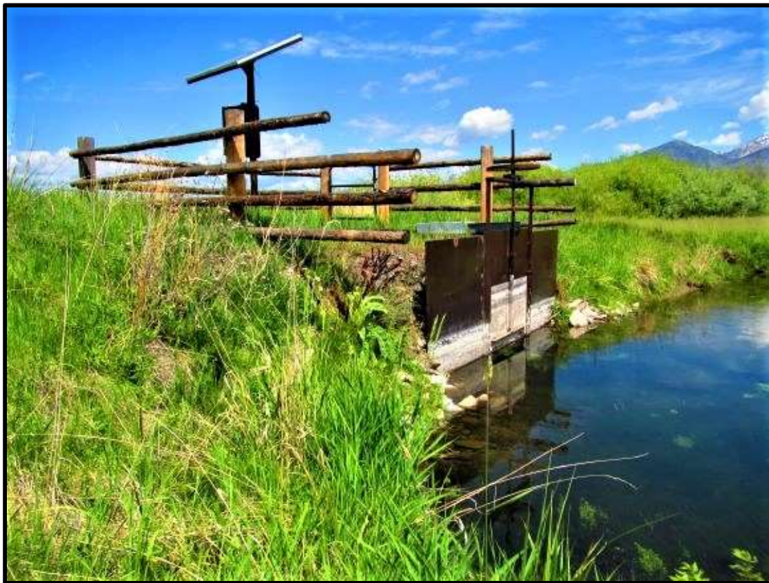
Photo 55. —The PBSC-10 fish screen was installed as part of a water savings, fish passage, and screening project.
