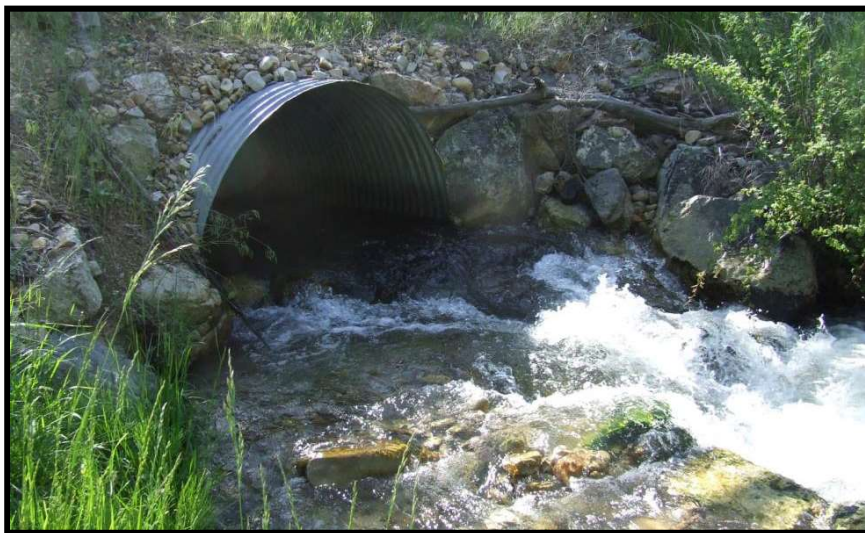
Photo 21. —Under-sized culvert on Sioux Lane across Tower Creek was a partial barrier to fish passage.
