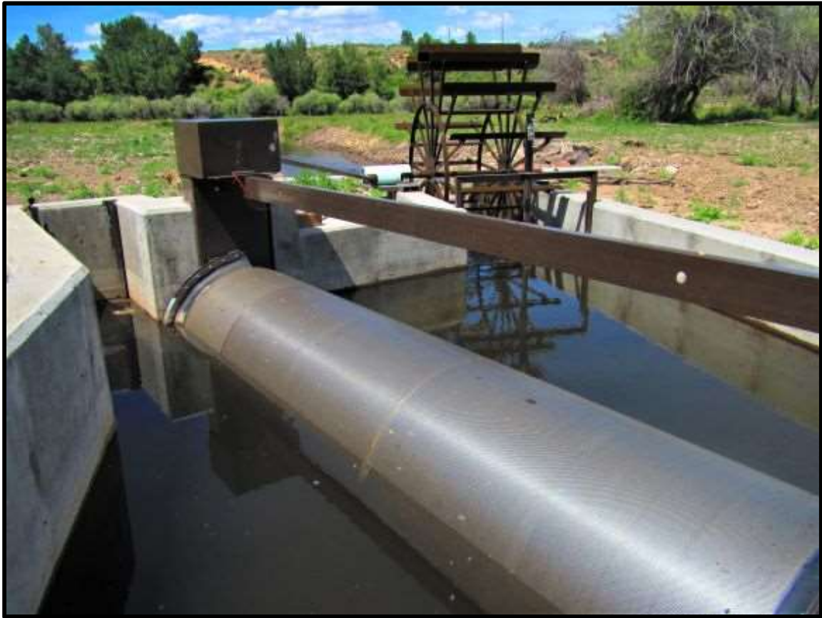
Photo 70. New NMFS Criteria fish screen installed at L-03AO is replacing a fish screen that was not functioning properly due to age and poor drainage.
