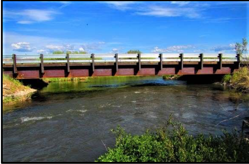
Photo 54. —New bridge across the Pahsimeroi River at Downton Lane was installed in 2016 to eliminate a passage barrier.
