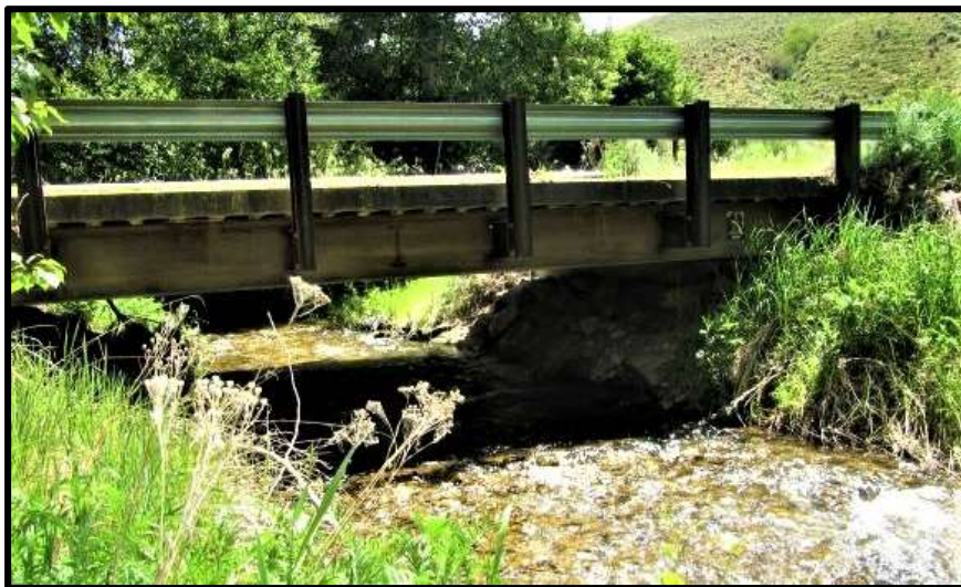
Photo 22. —New bridge across Tower Creek was installed in 2014 to eliminate passage barrier.
