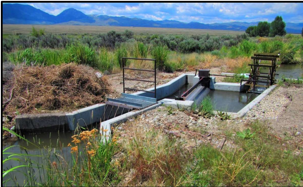
Photo 38. —The concrete and site were built for a NMFS criteria fish screen at the Pahsimeroi-16 diversion in 2015.
