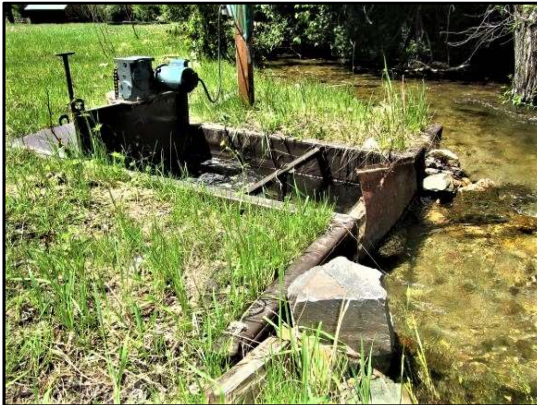
Photo 47. —New NMFS criteria fish screen installed at the Tower Creek-02 diversion in 2015
