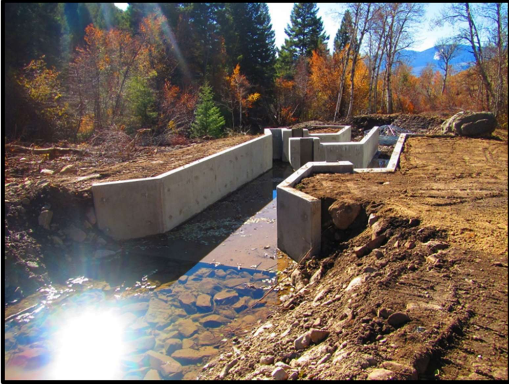
Photo 75. Pratt Creek-03 fish screen is ready for the screen components to be installed in the spring prior to irrigation season.
